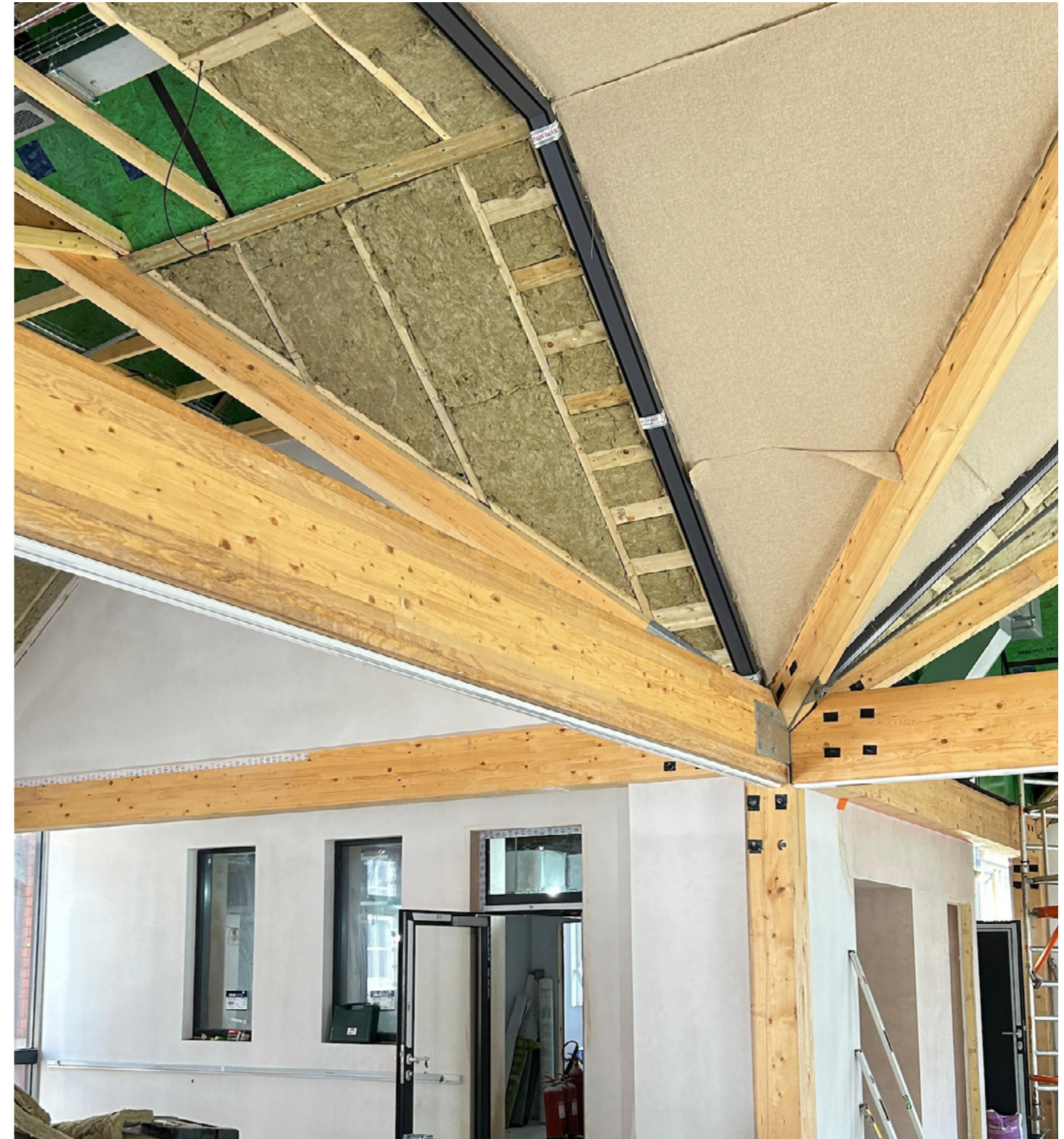
Figure 17. NMITE Skills Hub under construction - incorporating hybrid glulam beam combining softwood and hardwood. Photo: Michelle Gartside at Arbor Architects.
